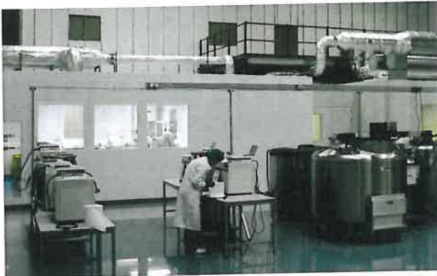
Stem cell laboratory with LN2 vessels and controlled-rate freezers prior to installation.
